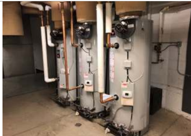
Photograph 99 Hot water tanks
