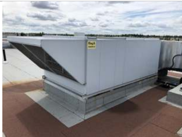
Photograph 116 Make-Up air unit
