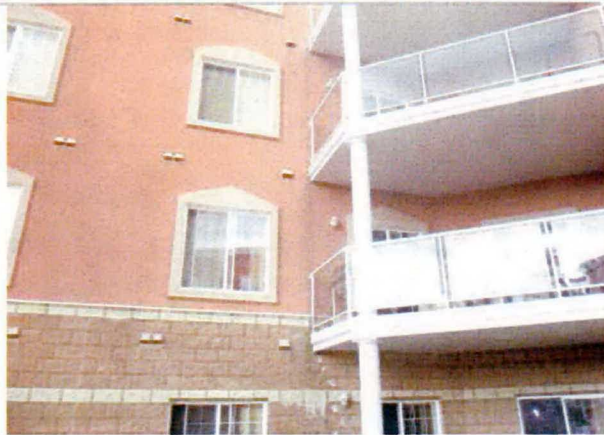
Staining on stucco below balcony to wall termination
