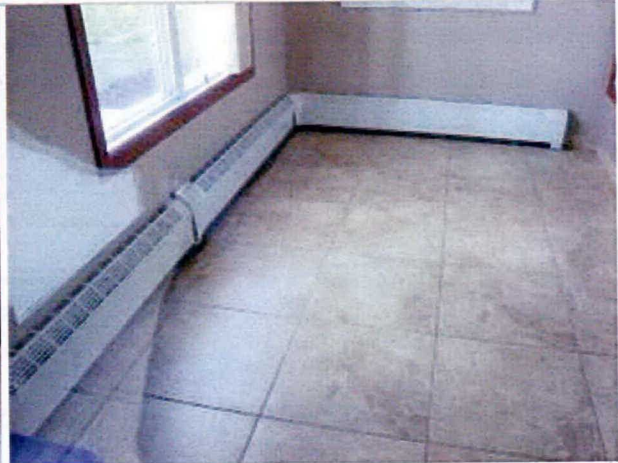
Baseboard heater in mailbox room
