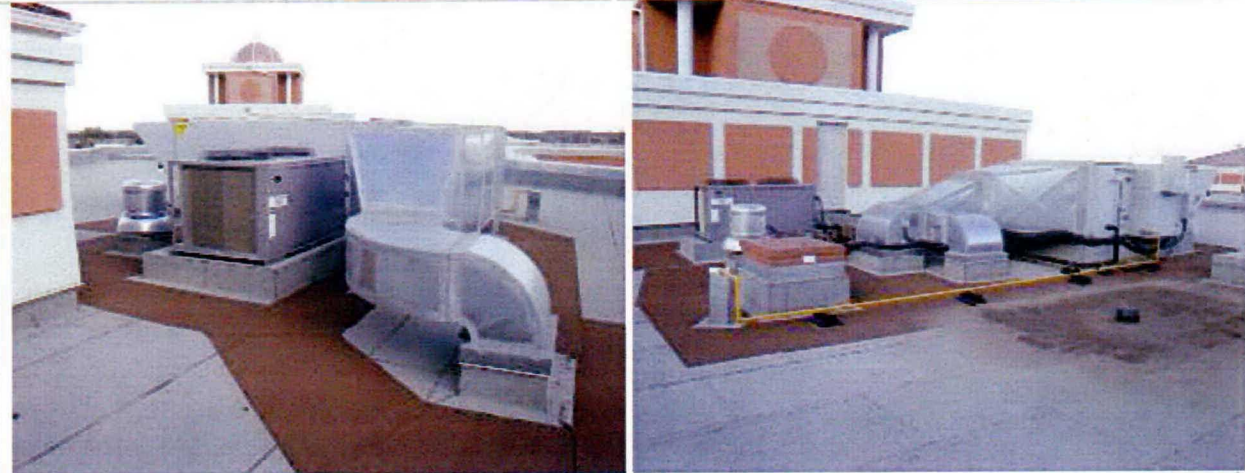
Make-up air units
