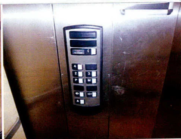
Elevator cab control panel
