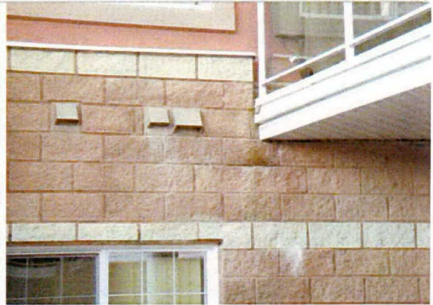
Staining on surface of architectural block below balcony
