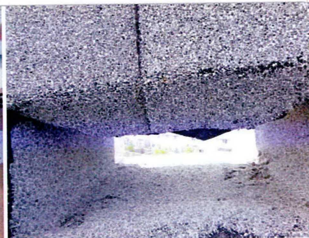
Incomplete detailing at overflow scupper drain
