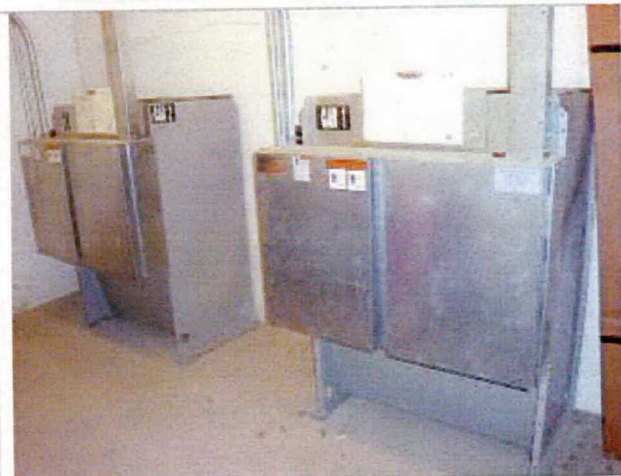
Elevator hydraulic reservoir and controls
