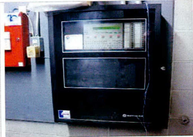
Main fire alarm
