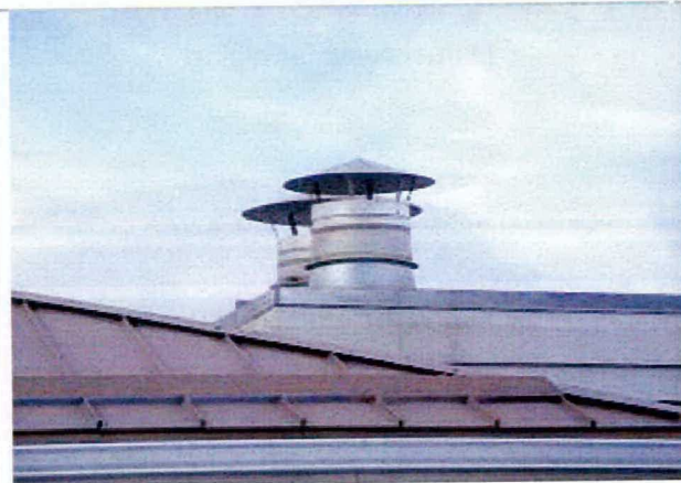
Boiler flue stacks
