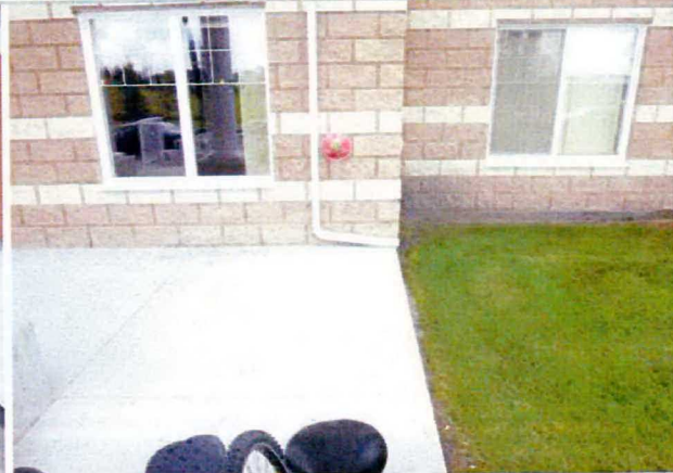
Downspout draining onto landscaping
