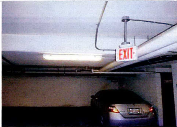
Fluorescent and exit lighting
