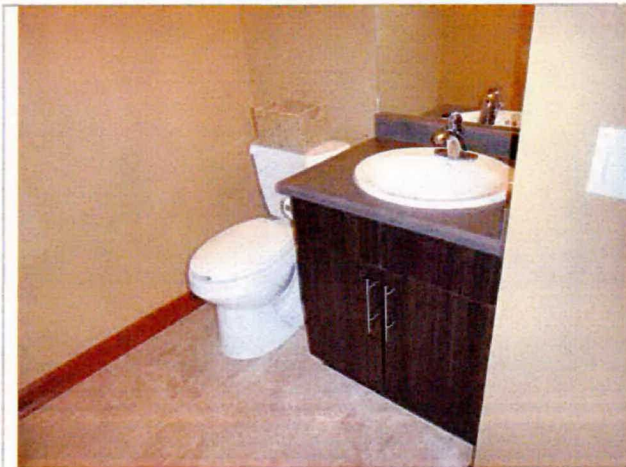
Plumbing fixtures in common room washroom
