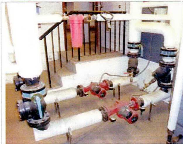
Heating supply pumps
