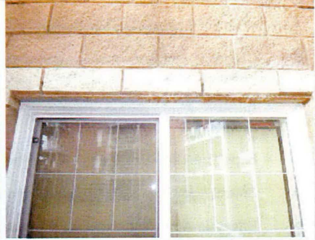
Corrosion on angle iron above window head
