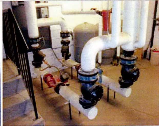
Heat loop piping and expansion tanks
