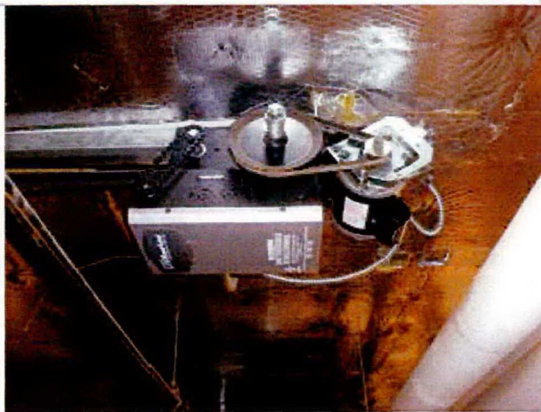
Parkade overhead door motor and controls
