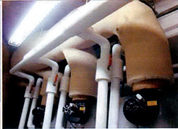
Domestic water piping
