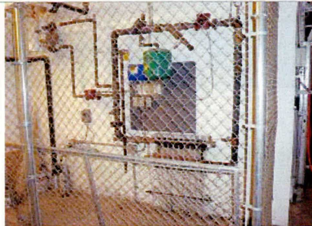
Parkade ramp heating system
